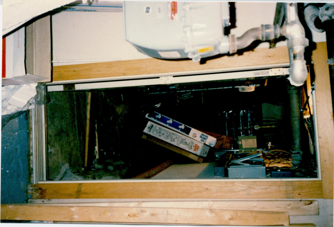
A-7 PHOTO OF THE UTILITY ROOM OFF OF ARCOMM'S STORAGE AREA. THE FRAMING WORK AROUND THE DOOR WAS BUILT BEFORE ARCOMM OCCUPIED THE OFFICE.
