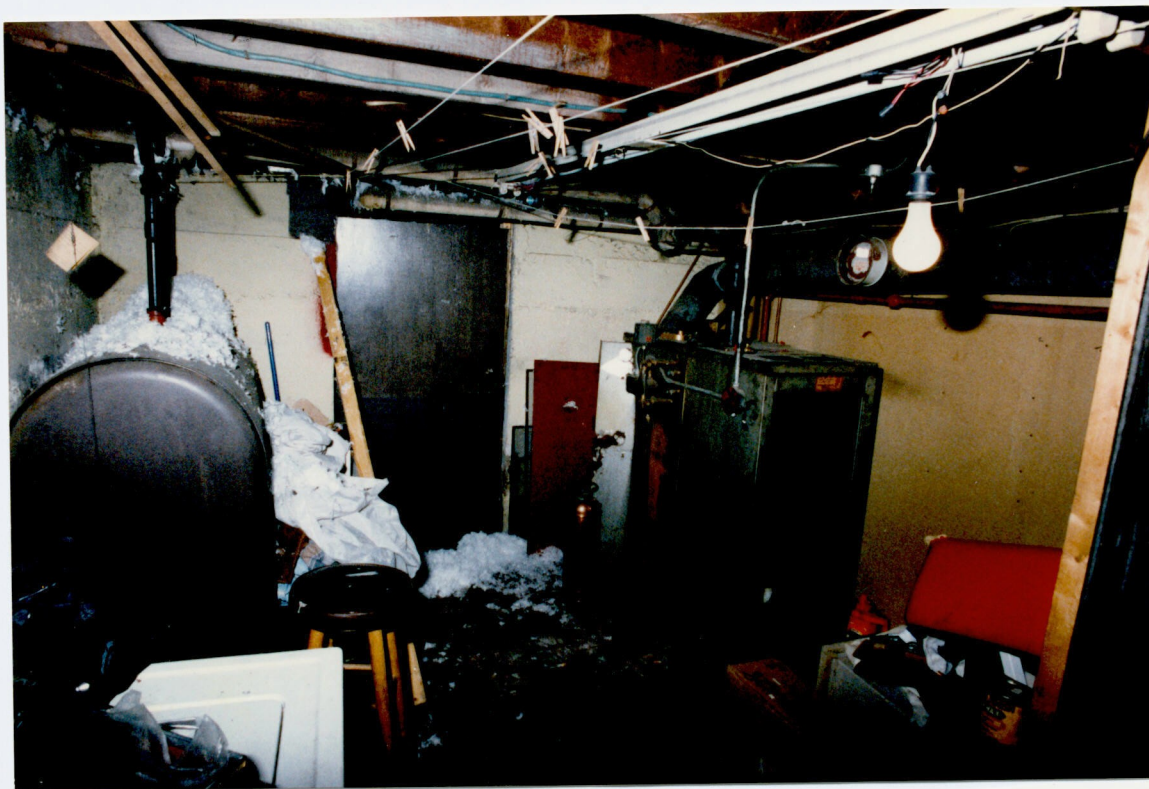
C-10 PHOTO OF THE COMMON AREA OF THE BASEMENT AS SEEN FROM THE BOTTOM OF THE STAIRWAY, LOOKING TOWARD THE FRONT OF THE HOUSE. THE DOOR IN THE PHOTO LEADS TO A STORAGE AREA UNDER THE FRONT OF THE HOUSE. THE WHITE SUBSTANCE OF THE FLOOR AND ON THE OIL TANK IS FROM THE EXCESS INSULATION THAT MIKE GREEN HAD INSTALLED IN THE HOUSE. TO THE RIGHT, NOT VISIBLE, IS THE ENTRANCE TO JOHN CATES APARTMENT.
